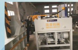
液压站油箱 Hydraulic oil tank
